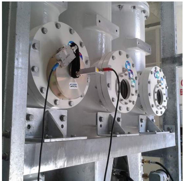
Example of UHF sensor fitting the circular dielectric glass window
